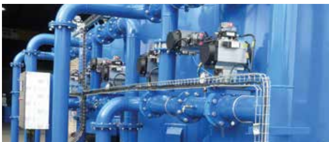
Typical side stream filtration plant ranging from 10 m 3 /hr to 400 m 3 /hr
