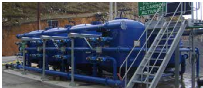
Side stream filtration designed and built for a plant in Peru, 8 vessels capable of filtering 800 m 3 /hr
