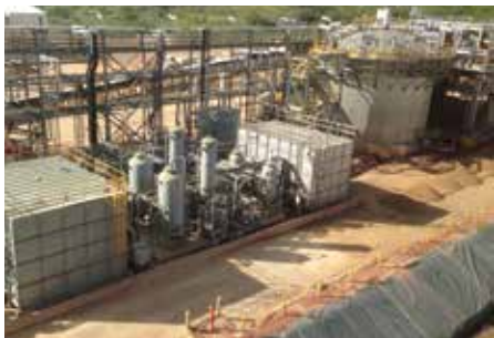
Demin water (45 m 3 /h), side stream filtration condensate polishing, potable water
