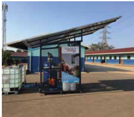
Containerised drinking water plant (Filtration, oxidation)
