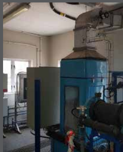
Pilot cooling tower
