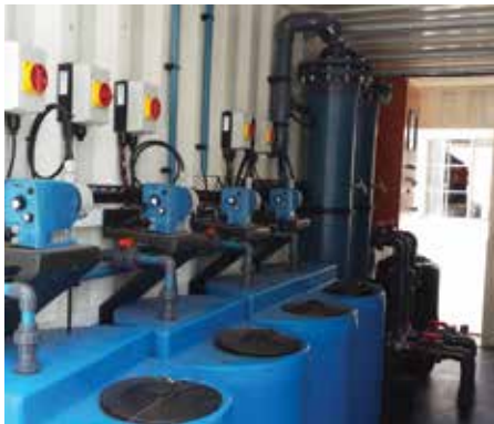
Dosing and control system
