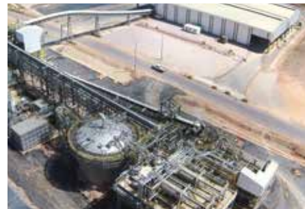
Treating surplus mine water to meet river discharge standards 5,2 million litres/day
