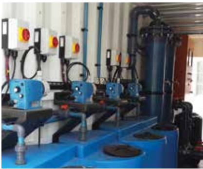
Dosing and control system
