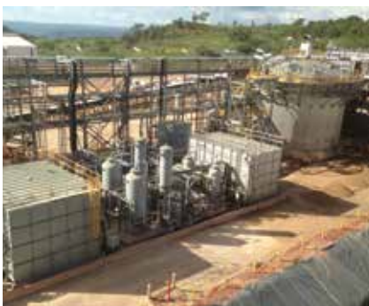
Demin water (45m 3 /h), slide stream filtration condensate polishing, potable water
