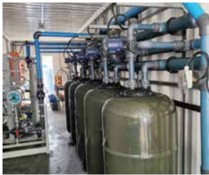
Containerised drinking water plant (filtration, oxidation)
