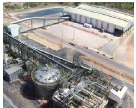
Treating surplus mine water to meet River discharge standards 5,2 million liters/day treated pre-oxidation – clarification – DM filtration – reverse osmosis
